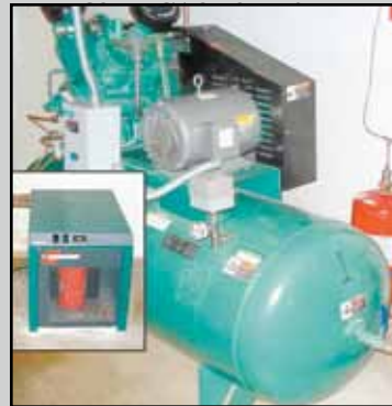
(1 OF 2) COMPRESSORS WITH DRYER
