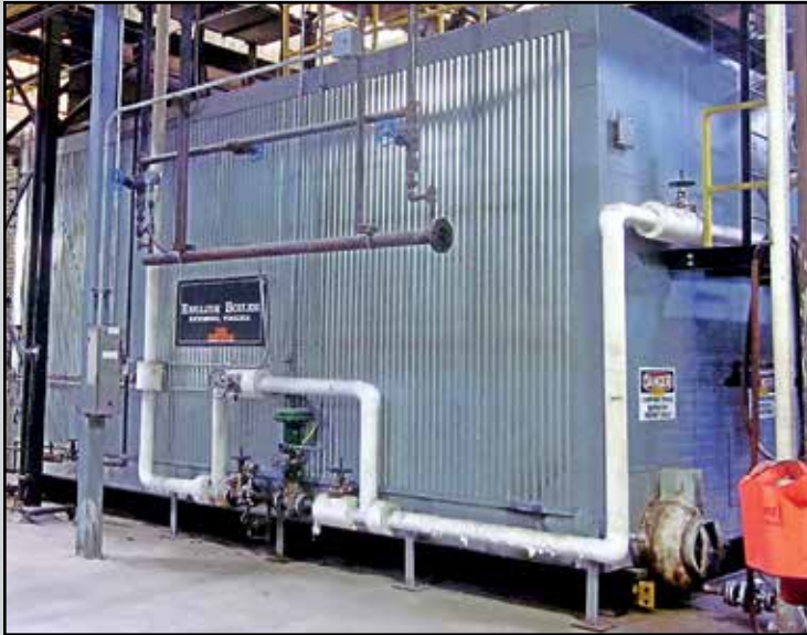
(1 OF 2) ENGLISH HIGH PRESSURE PACKAGE BOILERS
