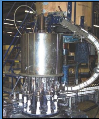
ELECTRONIC FILL LINE
