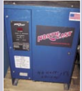
NORTHEAST 48V BATTERY CHARGER
