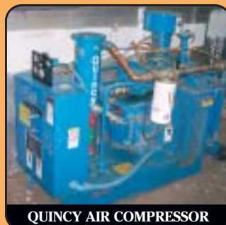
QUINCY AIR COMPRESSOR
