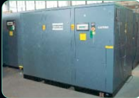
(1 OF 5) ATLAS COPCO COMPRESSORS
