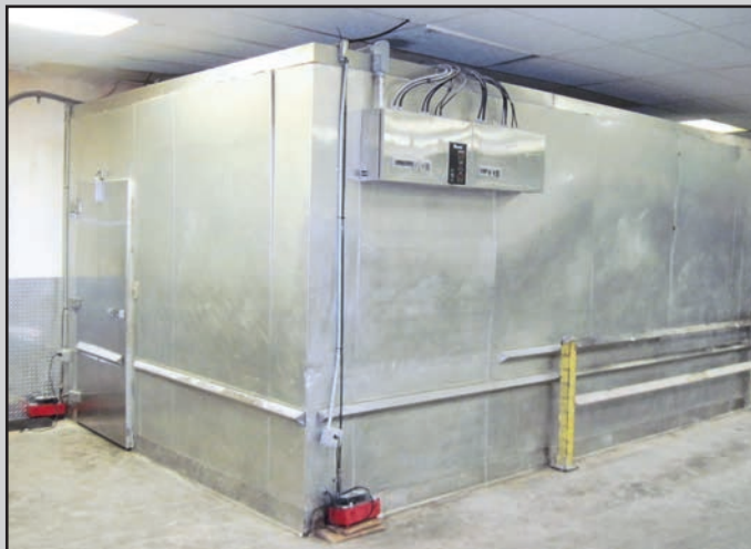
COOPER ROLL-IN PROOFER WITH REVENT CONTROLS
