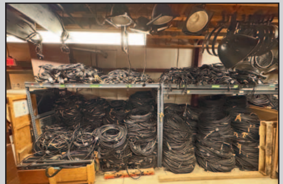
ASSORTED POWER CABLES
