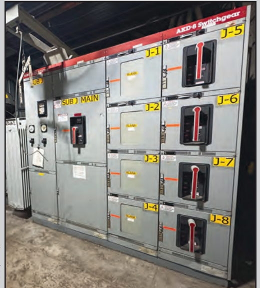
GE SUBSTATION TRANSFORMER WITH SWITCH GEAR
