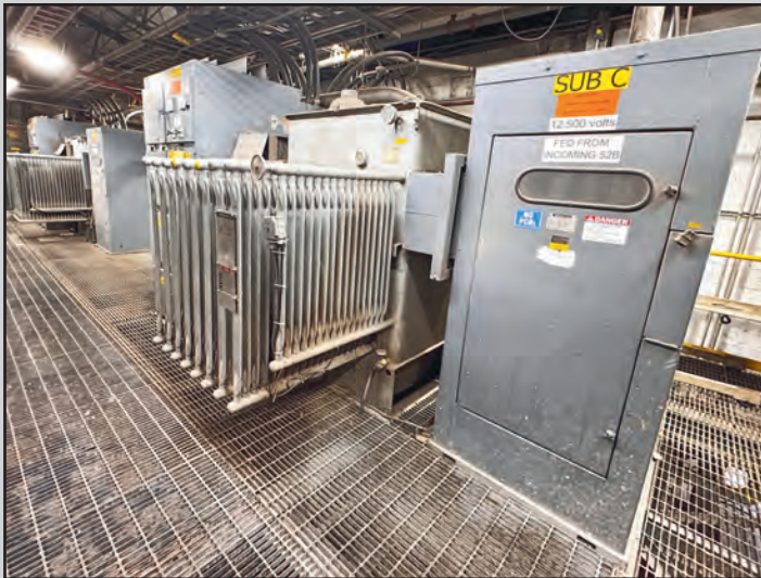
WESTINGHOUSE STEP DOWN TRANSFORMERS
