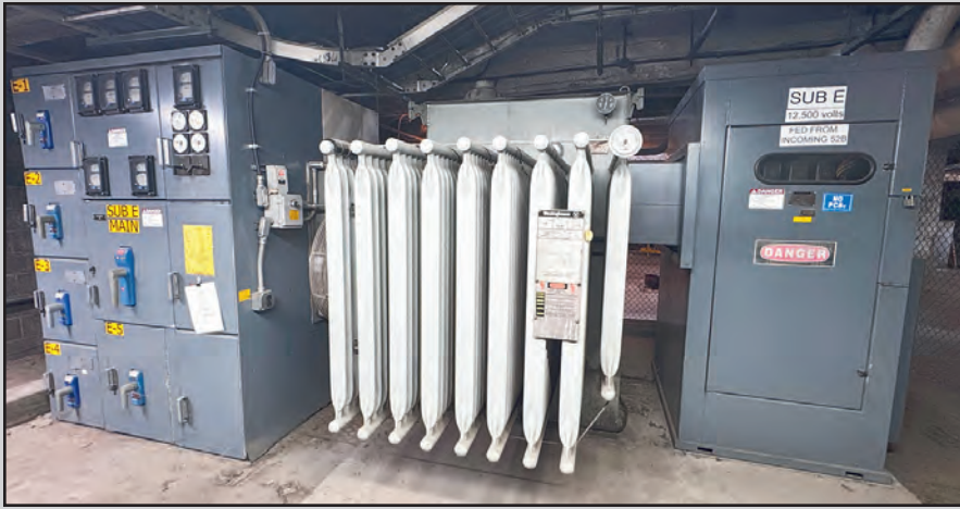
(1 OF 8) GE SUBSTATION TRANSFORMERS WITH SWITCH GEAR
