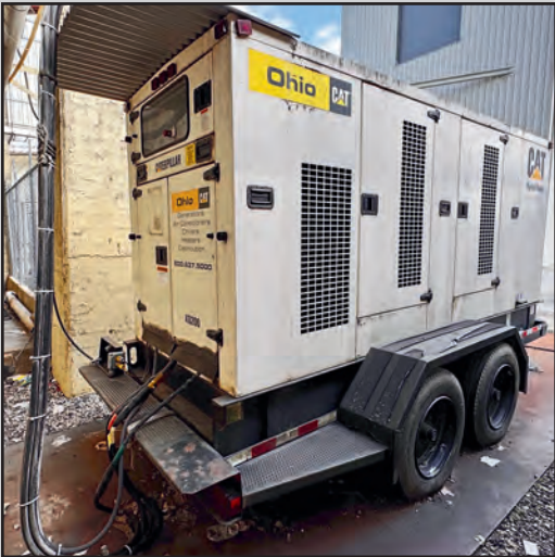
CAT XQ200 TOWABLE DIESEL BACKUP GENERATOR
