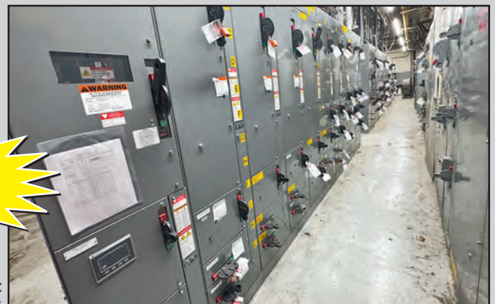
(SAMPLE) MCC SWITCH GEAR
