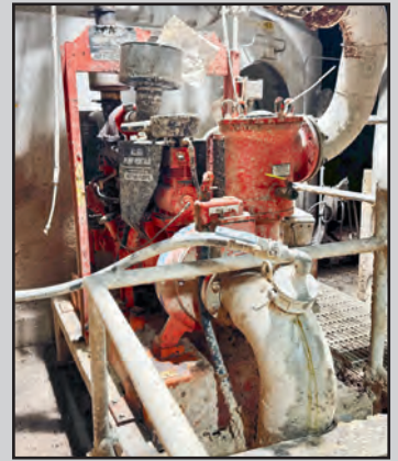
(1 OF 2) DIESEL 4" TRASH PUMPS
