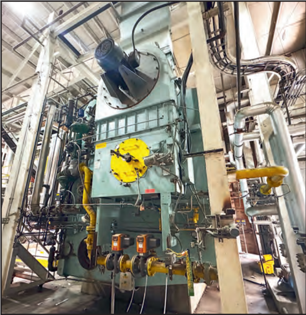
(1 OF 2) CLEAVER BROOKS GAS FIRED FIRETUBE BOILERS
