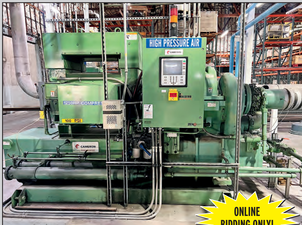
(1 OF 2) CAMERON 1,250 HP TURBO AIR COMPRESSORS
