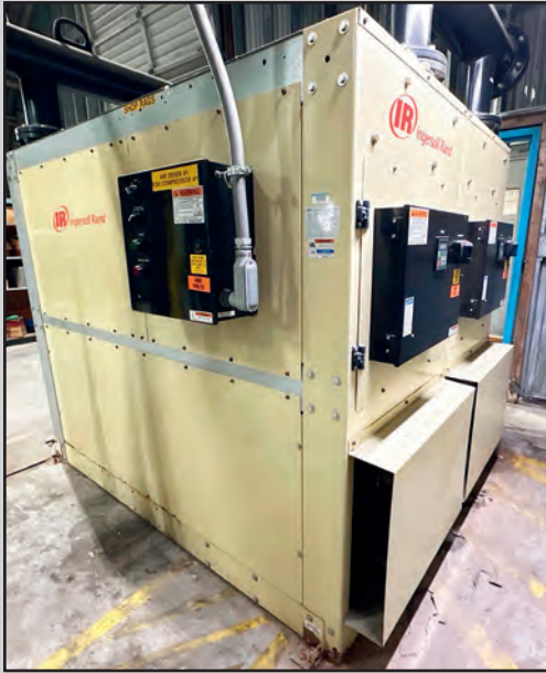
INGERSOLL RAND REFRIGERATED AIR DRYER
