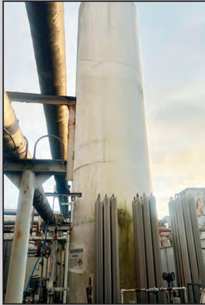
9,500-GALLON LIQUID NITROGEN TANK
