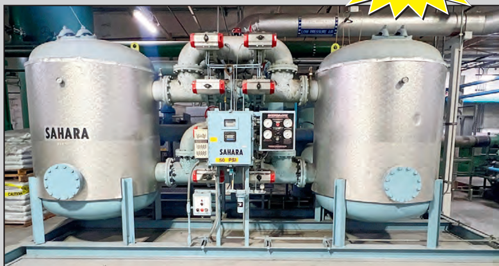
(1 OF 2) SAHARA DESICCANT AIR DRYERS
