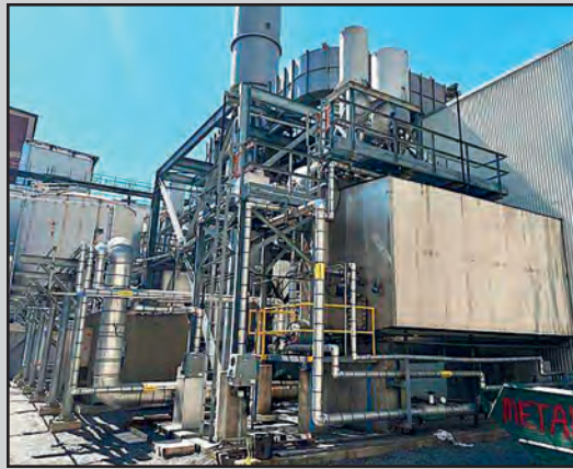
RENTECH PACKAGE STEAM BOILER
